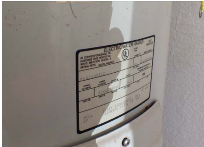
Water Heater MFG Date
