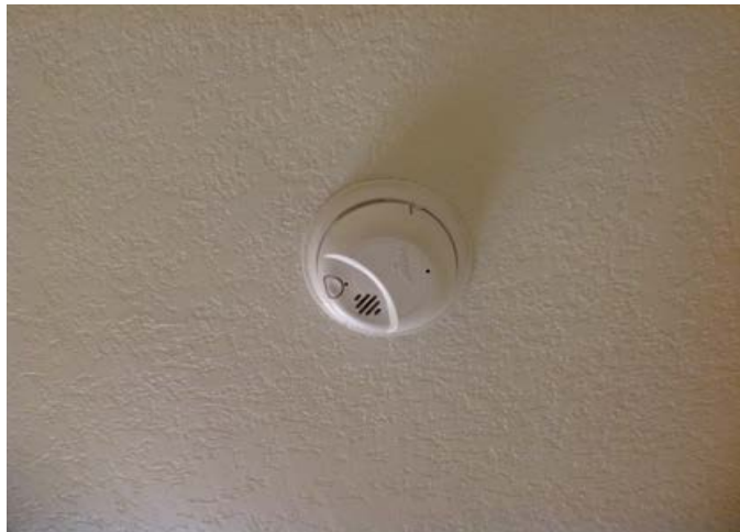
New Smoke Detector
