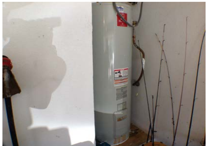
Water Heater(Gas or Electric)
