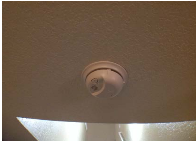
New Smoke Detector
