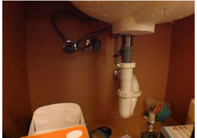
Cabinet Under Sink
