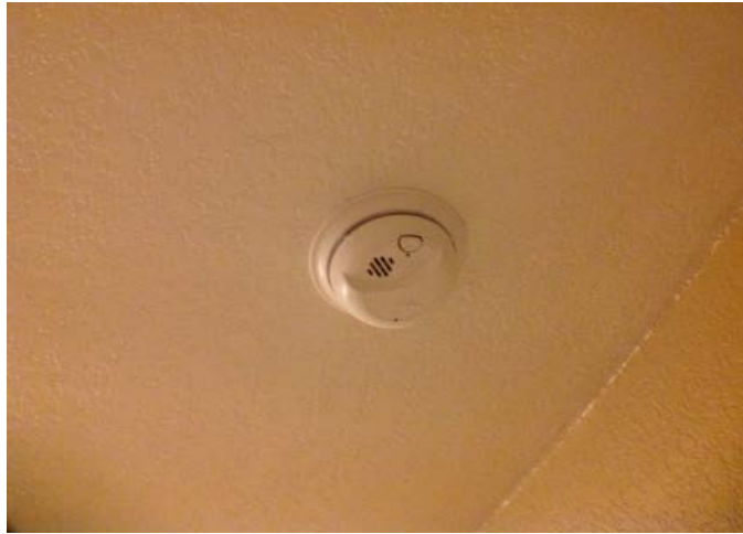
New Smoke Detector
