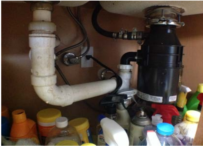
Cabinet Under Sink
