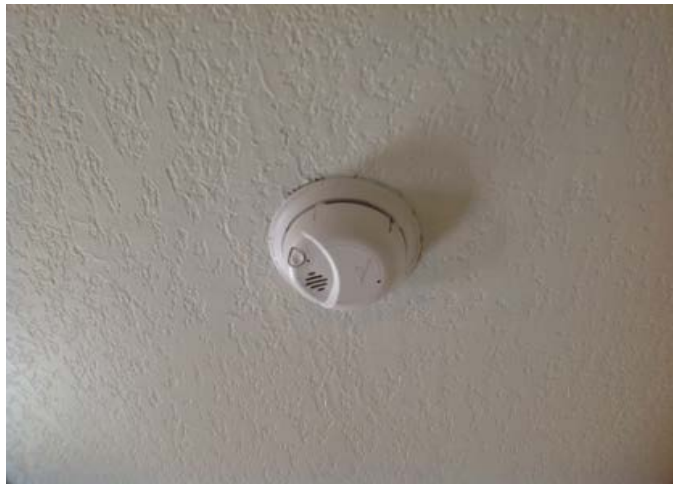
New Smoke Detector
