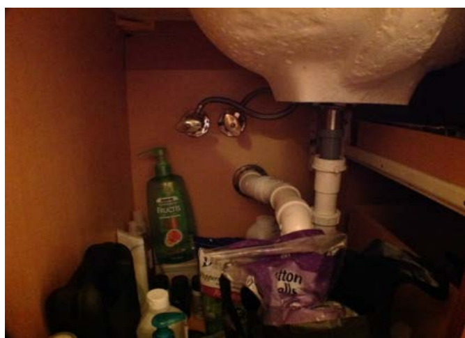
Cabinet Under Sink
