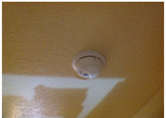
New Smoke Detector
