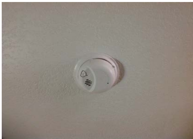
New Smoke Detector
